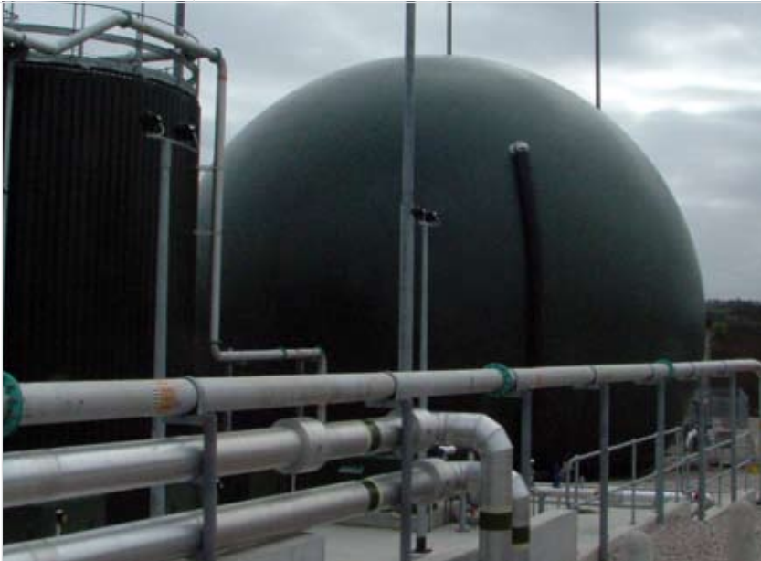
The digester stage is made more efficient and effective, cutting 99% of pathogens from the sludge
