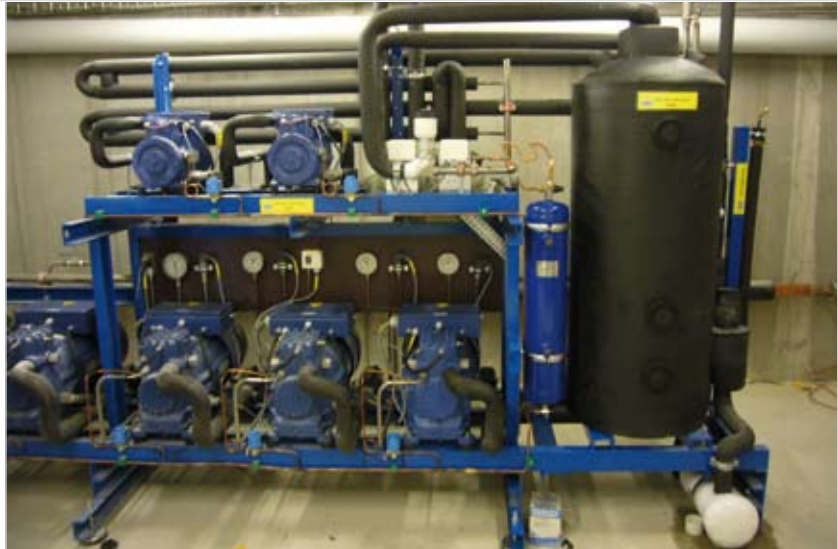
The CO 2 Ref compressor system installed at the Roskilde supermarket
