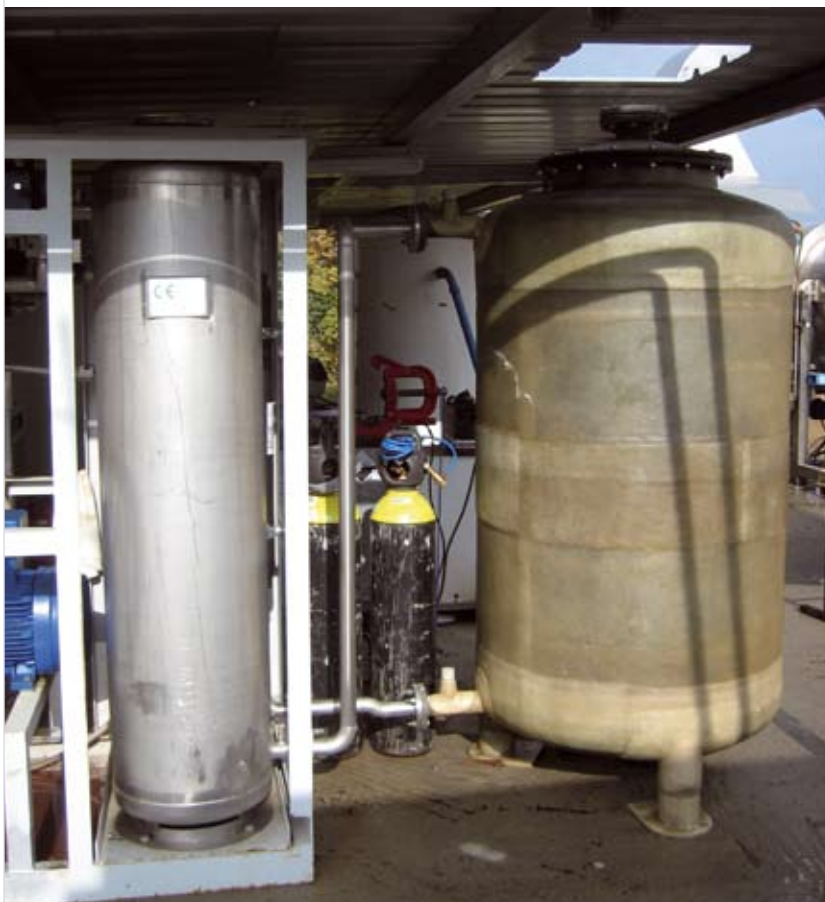
Biogas was upgraded with the use of biofilters and an activated carbon filter, which removed hydrogen sulphide ( H_2S ) and siloxanes
