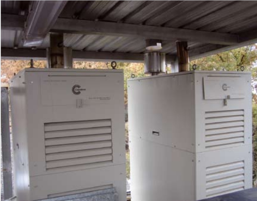
Two 30 kW microturbines were installed on the Orís landfill and operated successfully with gases with methane levels of 35% or lower
